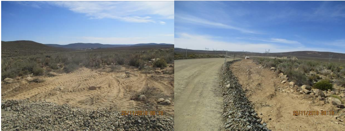
Photos: Damaged area used as a turning point by graders, excavators during preparation of culverts and V-drain require rehabilitation.
